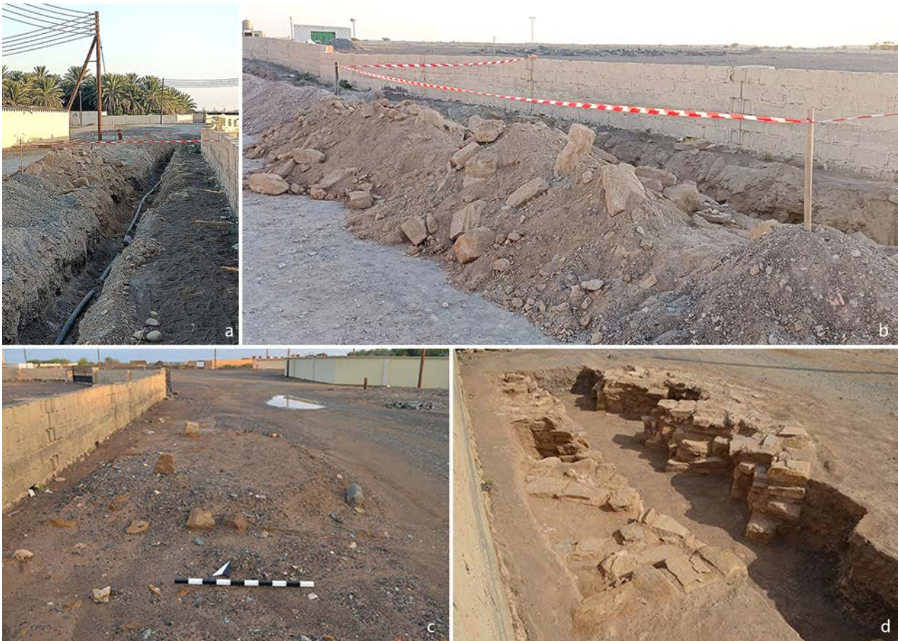
Figure 1. Umm an-Nar period tomb in Al-Musalla: a-b: construction of water pipe in Al-Musalla 2022, which accidentally hit an Umm an-Nar period tomb (photos: Abdallah Al-Amri); c: tomb before excavation, and d: tomb after excavation in 2024.
