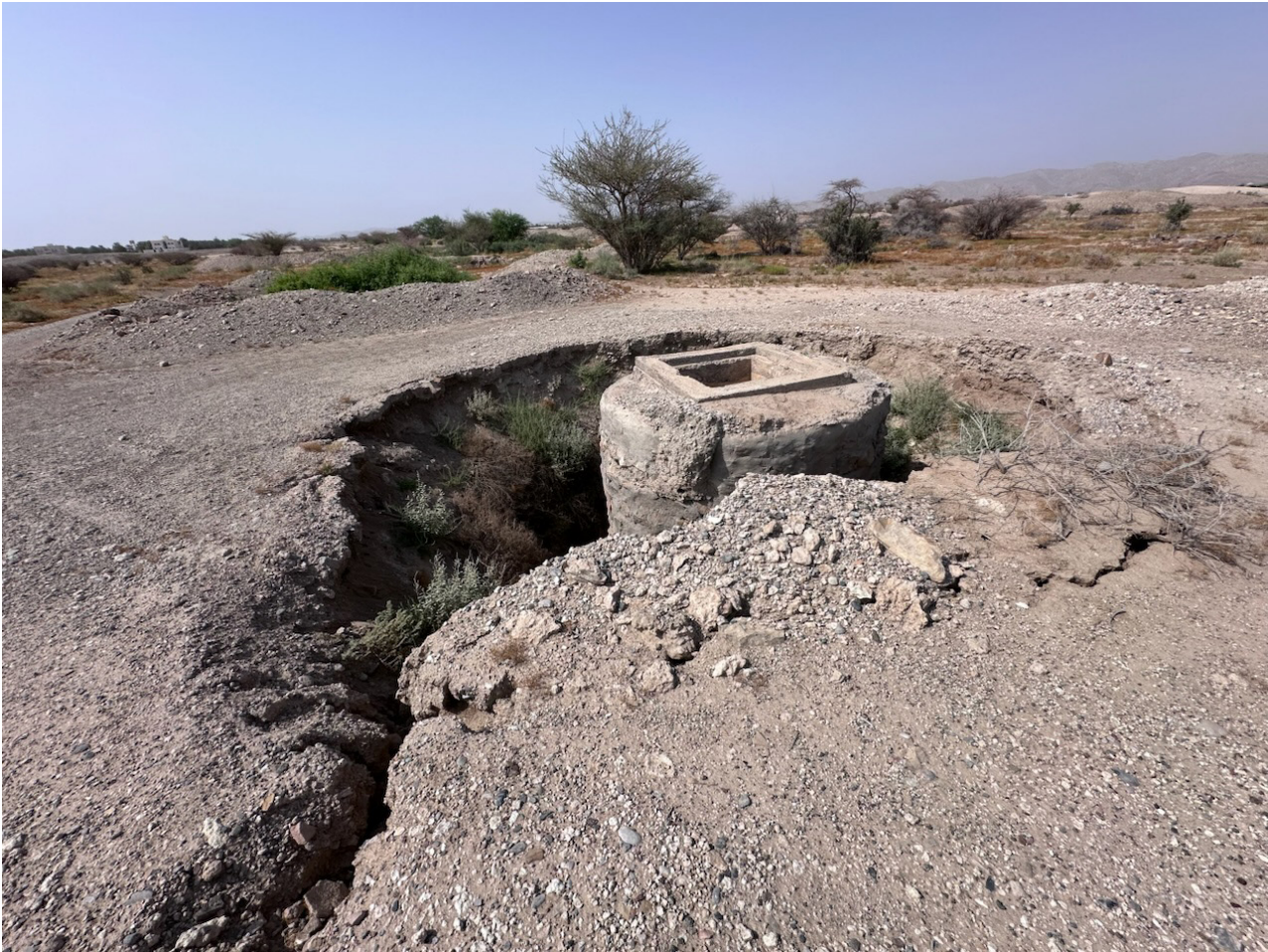
Figure 7. The shaft of a falaj exposed by the 2024 strong rainfall.
