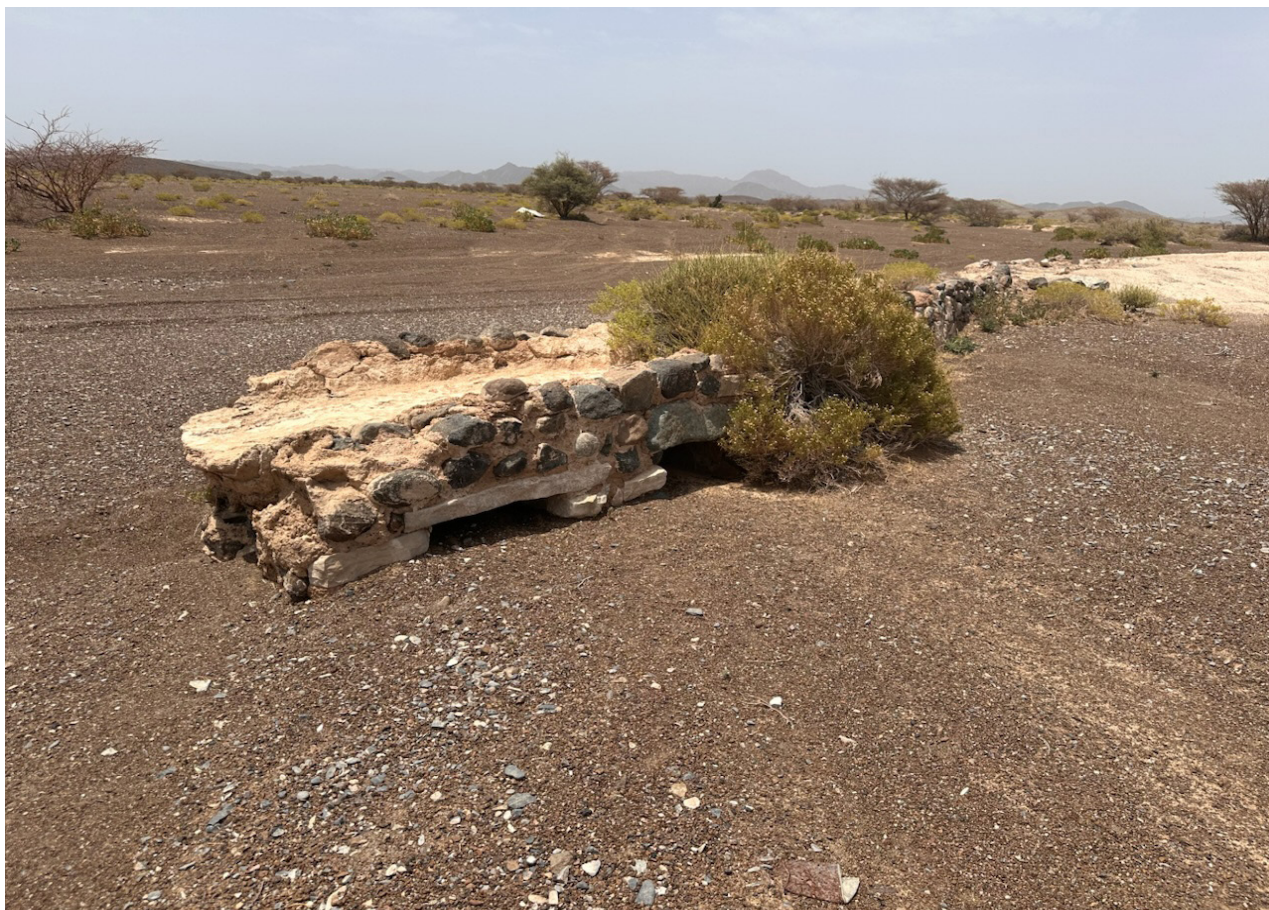
Figure 6. A surface canal damaged by floods.
